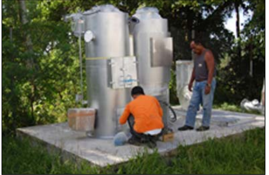
Incinerator on site at Chuuk State Hospital
